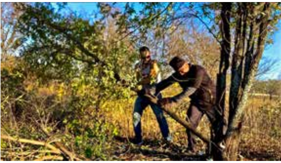
Clearing hackberry tree overgrowth, Fort Worth Prairie Park, Richardson Tract - Benbrook Lake / U.S. Army Corps of Engineers / Great Plains Restoration Council / Restoration Not Incarceration™
